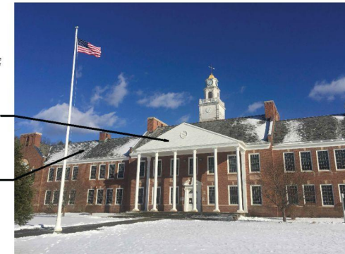
Photo shows prior changes to original construction and demonstrates the continued deterioration of the cupola. Photo ca. 2018
